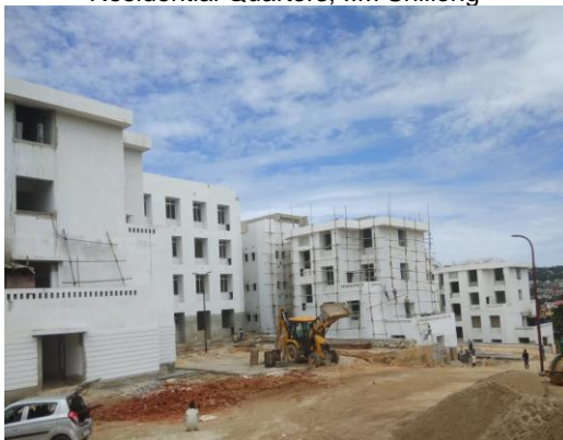
Construction of Office cum Laboratory Complex including Regional Training Institute of Geological Survey of India, NER at Shillong
