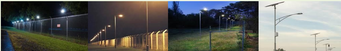
Different examples of Perimeter lighting
