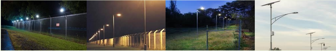
Different examples of Perimeter lighting
