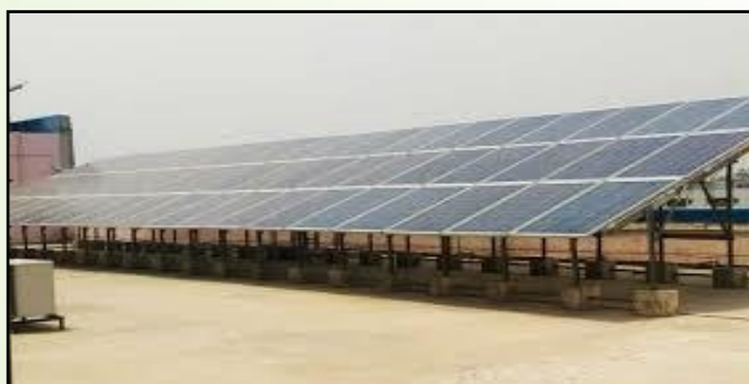
FIG 4. SOLAR PANELS AT GOVT. BUILDING SOURCE : SAURENERGY.COM)
