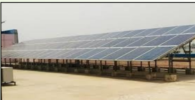
FIG 4. SOLAR PANELS AT GOVT. BUILDING SOURCE : SAURENERGY.COM)
