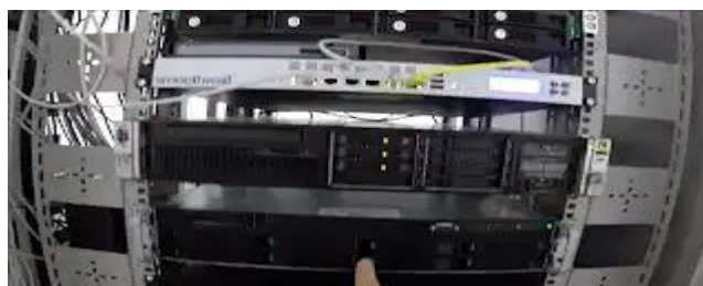
Figure 37: View of Active Rack
