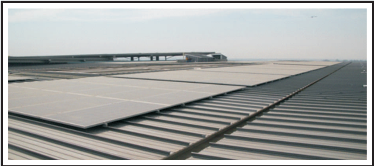
200 KWp Rooftop Solar Panel at PNB Headquarter Building, Dwarka, New Delhi
