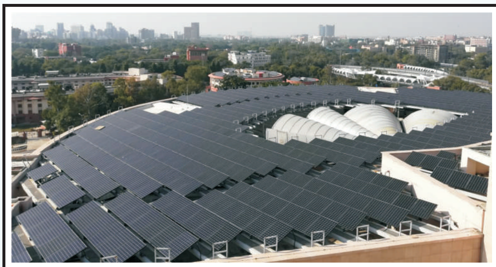
1400KWp capacity Solar Panels installed at Additional Office complex for supreme court, New Delhi
