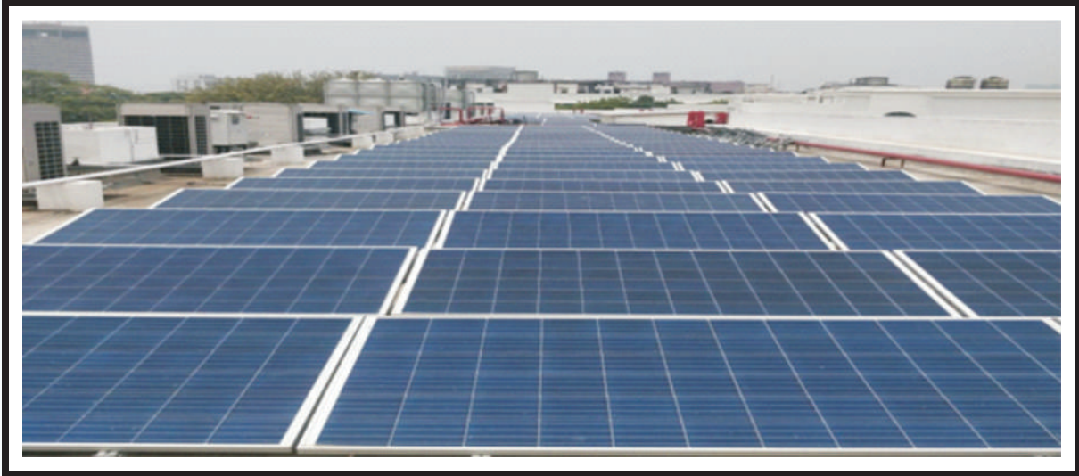
75 KWp at Western Court Annexe Building at Janpath, New Delhi
