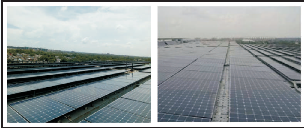
Bird's Eye view of Solar Panels on Indira Prayavaran Bhawan, New Delhi – Capacity 930 KWp.
